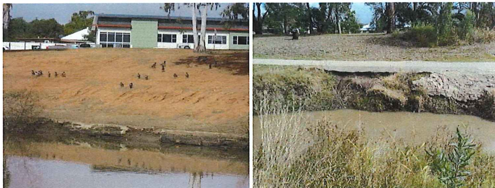
Plate 9 Erosion at Shadys Lagoon (Site 3a left) and Bungil Creek (Site 3c right)
